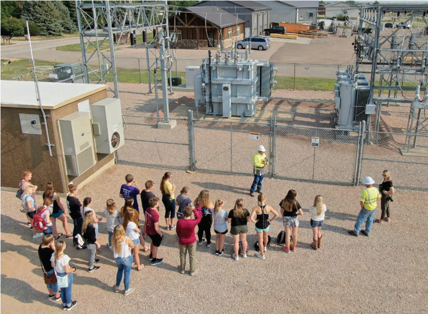
Dozens of high school students from across South Dakota took part in a youth leadership experience sponsored by South Dakota electric cooperatives. As part of the event, attendees learned about electric power production (pictured above).
