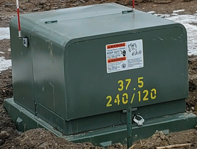
"Green boxes" are a critical part of the power delivery system used by your co-op. Photo by Journey Lineworker Mike Oines
