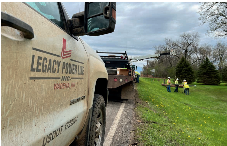
Left: Legacy Powerline Inc., of Wadena, Minnesota, is one of several overhead power line construction contractors used by Sioux Valley Energy in recent years. Top: Friest Tree Experts is one contractor the Cooperative uses. The Harrisburg, S.D., company specializes in trimming trees around power lines. Above: Bruce Barrick and Tim Fey comprise SVE's Contractor Relations Department.
